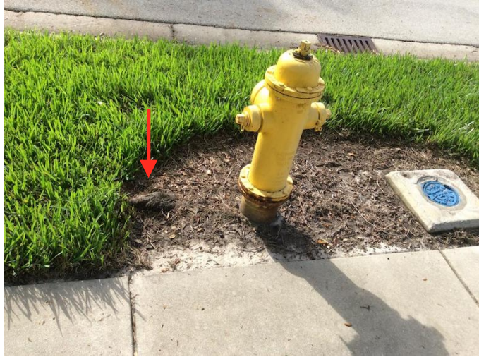
Image 22. A tree root approximately 4 inches in diameter impacting a fire hydrant.
