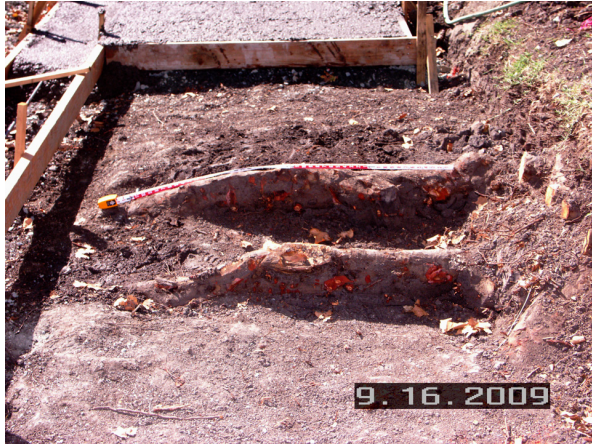
Image 13. Prior to plate installation, two 4 to 5-inch roots were retained, bruised a bit by the construction crew who did this by hand. Notice smaller roots at the surface were cut.
