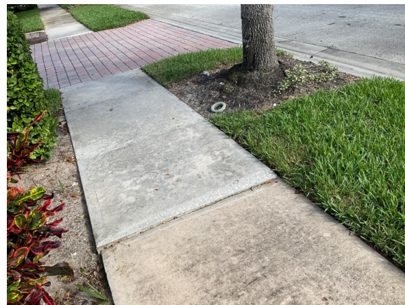
Image 3. Tree #461. Supportive lateral roots were cut to install a new sidewalk slab. This temporary fix, which has failed allowing the new roots to lift the replacement sidewalk, has also destabilized the tree.
