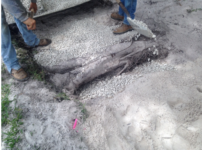
Image 9. Level the soil around the excavated root. The resulting sidewalk may be higher than the old sidewalk.
