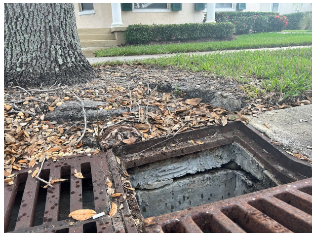
Image 18. A tree root is seen growing between and slowly separating the spaces in the engineered valley gutter.
