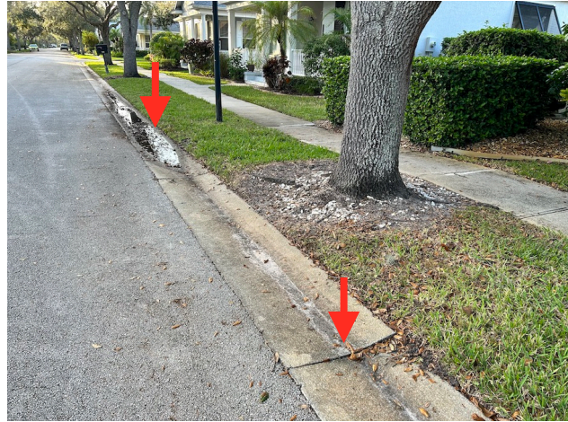
Image 17. Valley gutter function is hindered as a result of impacts by tree roots. Arrows indicate lifted valley gutter and pooling water.
