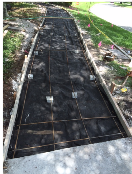
Image 12. Geotextile fabric is then laid over the #57 stone and geogrid mat and rebar reinforcement is then installed over the geotextile fabric.
