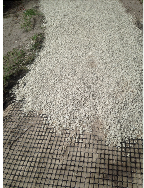
Image 10. Install geogrid mat over the roots and cover the geogrid mat with #57 stone.
