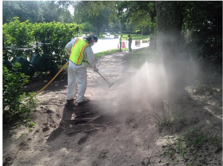
Image 6. Use an air excavation tool such as an Air Spade or Air Knife to locate roots and remove soil from roots. Hand digging is also possible but roots can be damaged.
